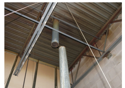
The broken stove pipe.
