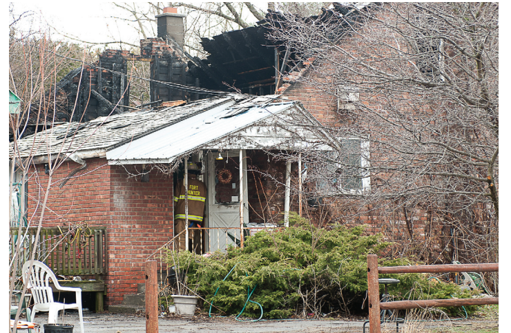
A blaze which started during the early morning hours of Tues., April 4, destroyed this home at 2973 Curry Road in Guilderland.
