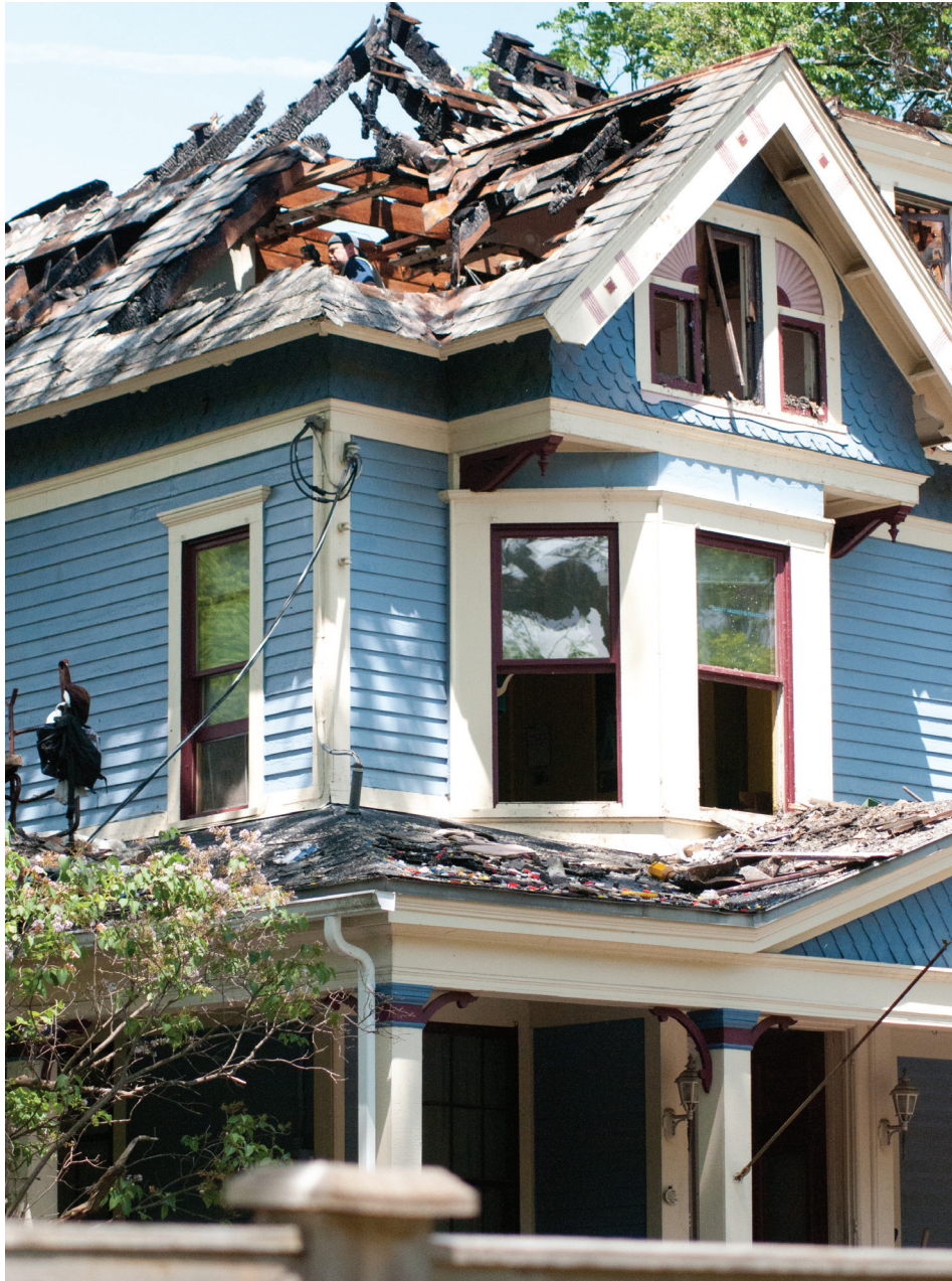
The roof is all but gone from the historic Slingerlands home on the morning following a late night fire. All four family members escaped harm. Photo by Michael Hallisey / Spotlight News
