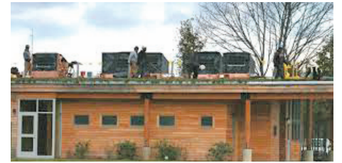
Contractors install the green roof on the new Five Rivers Visitor Center.
