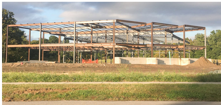
The 26,000-square foot construction site, above, remains incomplete; it could still go untouched for months.
