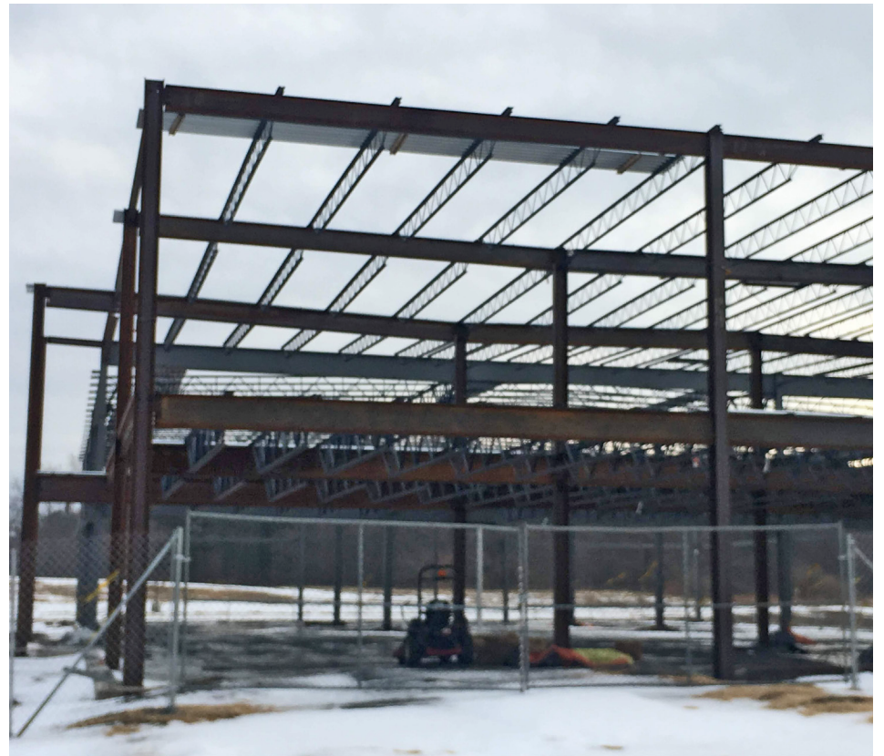
A chain linked fence was installed two weeks ago to surround Monolith Solar's incomplete Slingerlands headquarters construction site.
