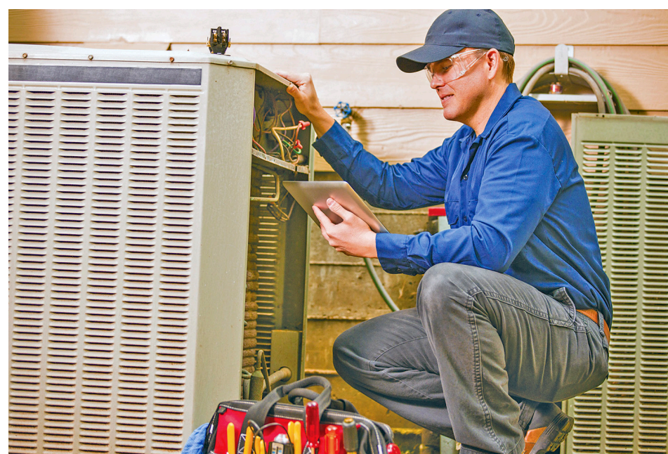
Periodic maintenance of an AC unit will keep it in good repair and working efficiently.
