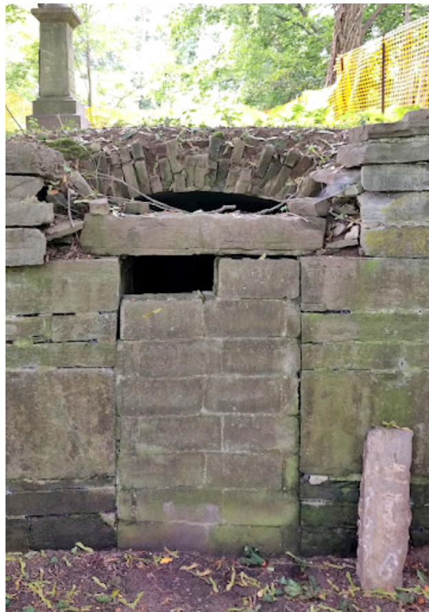
The Slingerland Family Burial Vault sits within a hillside near the New Scotland and Kenwood avenue intersection. Its current state is the result of many years of neglect.
