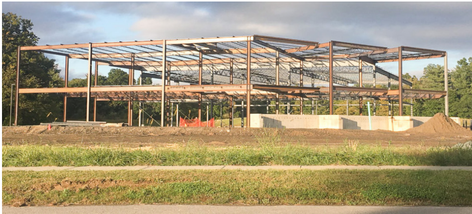
The construction site of the company's Slingerlands headquarters building has been on pause for almost a year now and it is unknown whether it would move forward.
