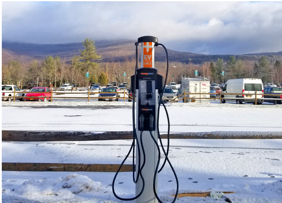
The five potential electric vehicle charging stations that the public can use once they are installed at three lots on Bethlehem town property will look like the one above.
