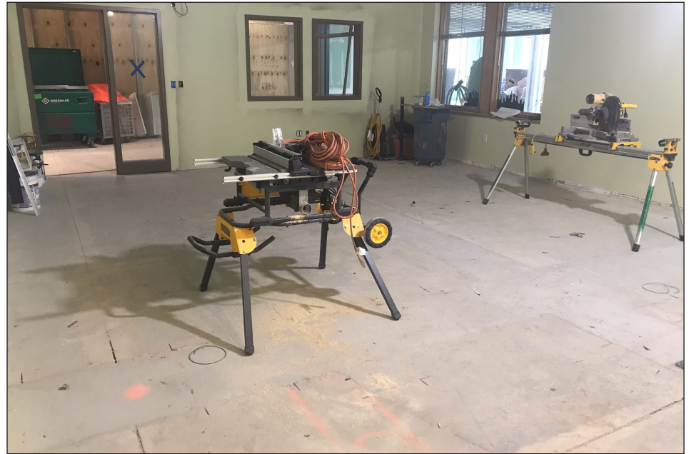
Guilderland Public Library is constructing a dedicated teen room as part of its building project, which is roughly halfway done. About 70 percent of the library's interior is currently closed off for construction. This project is expected to take one year, with completion anticipated for this fall.
