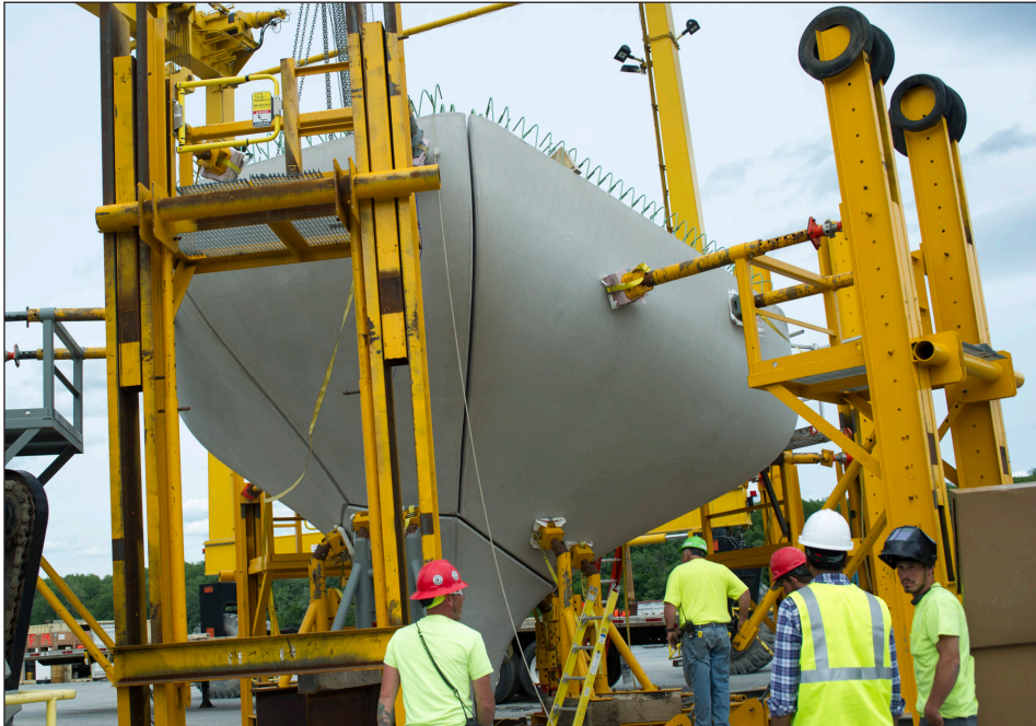
Port of Coeymans becomes the second construction hub for the Sunrise Wind project.
