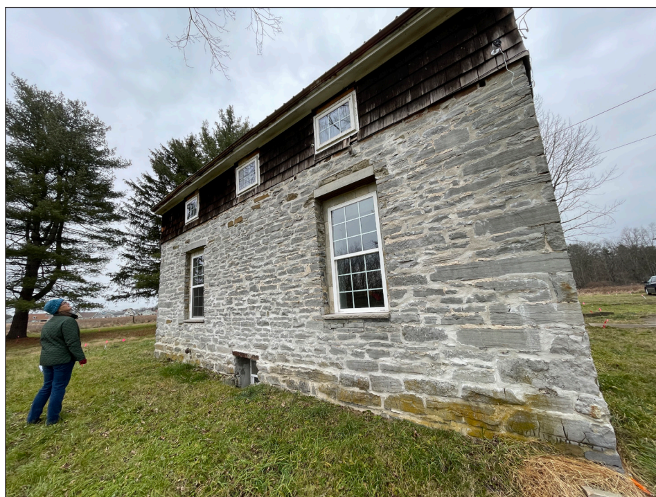
Bethlehem Town Historian Susan Leath peers up towards the pitched roof of 246 Van Dyke Road, otherwise known as the Bradt-Oliver House. Now a patchwork of construction that shows both its original structure incorporated with 20th century woodwork, the home appears on the town's earliest of maps from the 18th century. Otherwise, it is not clear when it was first built. On the 1767 map, on which it is referenced, the Bradt family is listed as the owner. It was a Bradt after whom the Normanskill was named.
