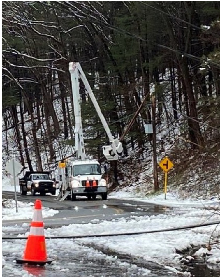
A National Grid crew works on freeing a powerline from surrounding trees after an early spring snowstorm dumped more than a foot of snow in the hilltowns last week, knocking out power to thousands.
