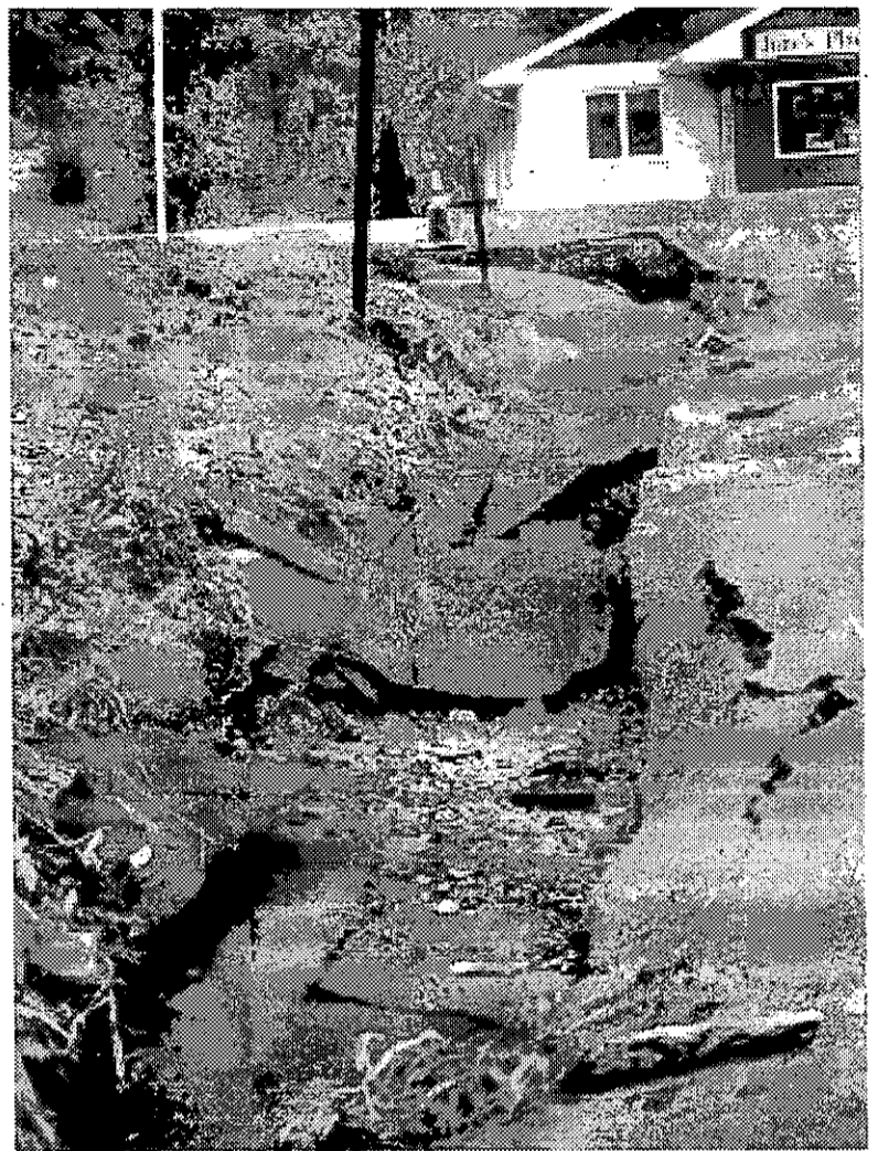
A portion of Mill Road in Clarksville washed away near the Bell home.
