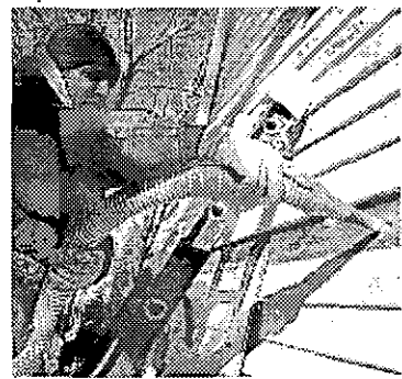
Certified Home Performance Contractors install cellulose made of ground-up newspapers and a fire retardant to increase insulation.
