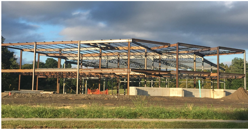
Monolith Solar has suspended construction on its new headquarters in Vista Technology Campus in Slingerlands.
