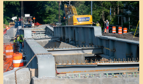
Crews begin the emergency removal of the new County Rail Trail bridge over Route 85 in Slingerlands that collapsed last week. The County is planning to put a temporary span in its place until a new bridge can be designed and fabricated.
