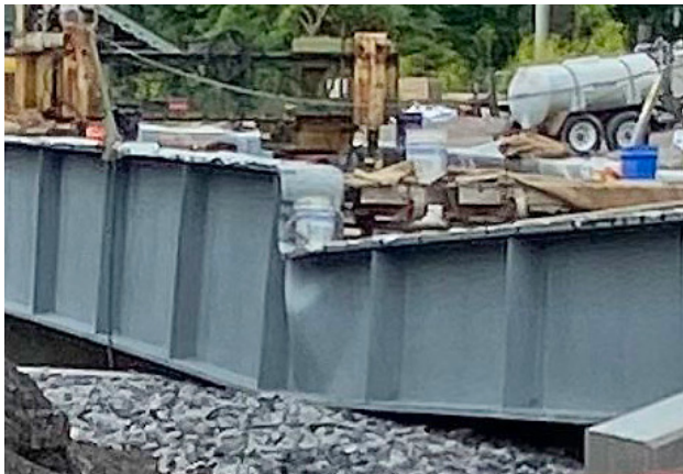
The transition point where the new bridge buckled. Photo by Scott Anson
